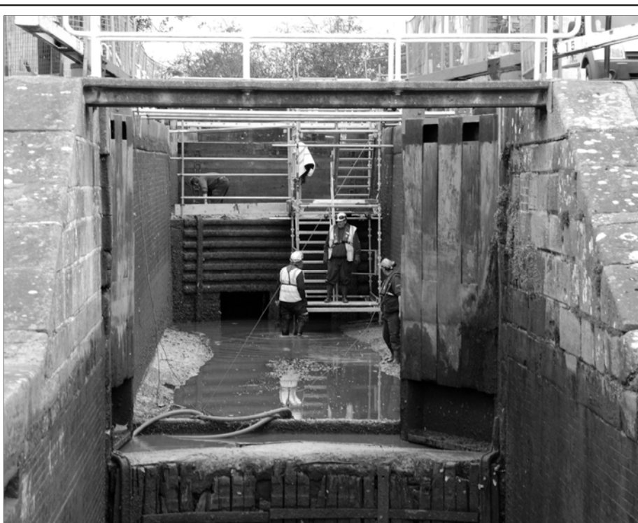
This is an unusual view of Bunbury Locks taken in November. The lock was drained for maintenance work, exposing the original construction and timbers. It would be interesting to know if any treasure was found at the bottom.
